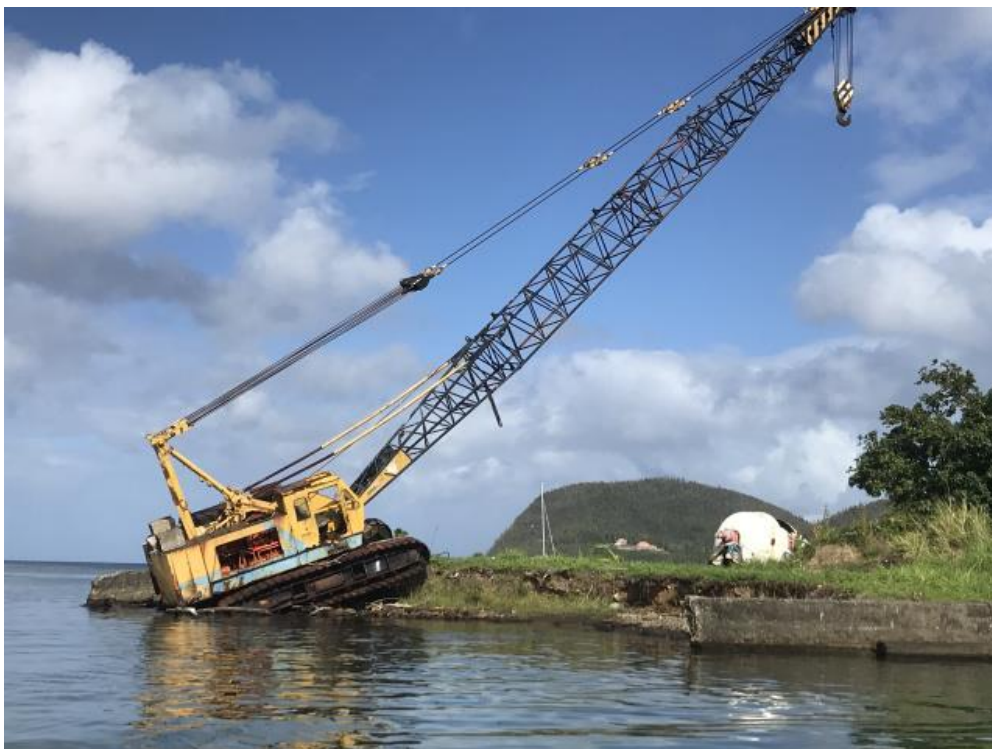
Hurricane damage from Maria in September 2017. Many of the buildings in Portsmouth were still uninhabitable
