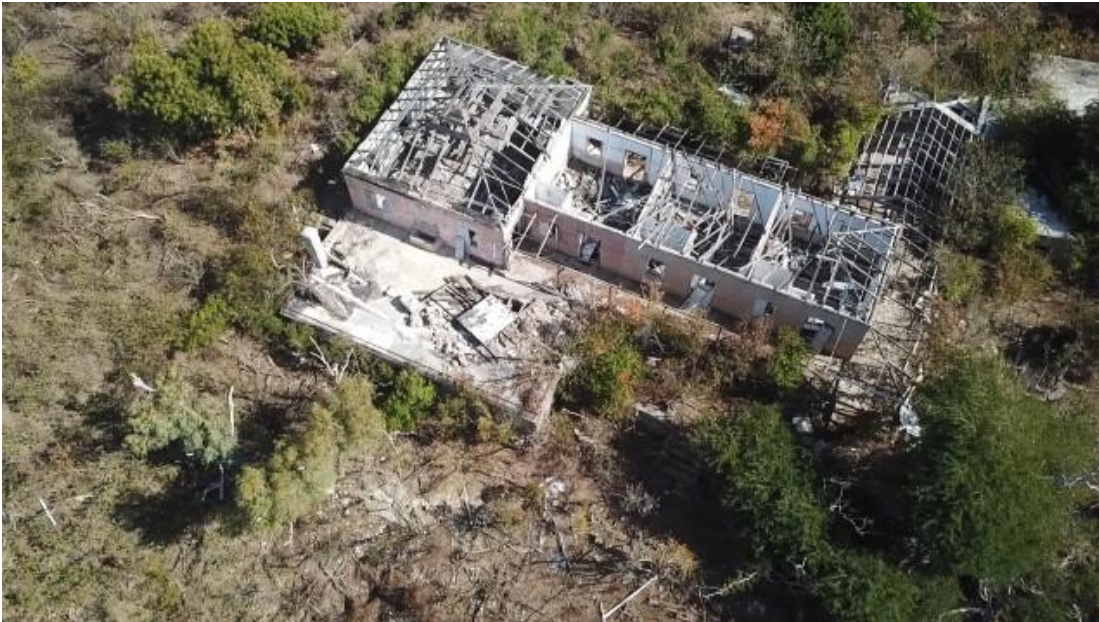
This used to be a nice house on the tip of Peter Island...as seen by the drone
